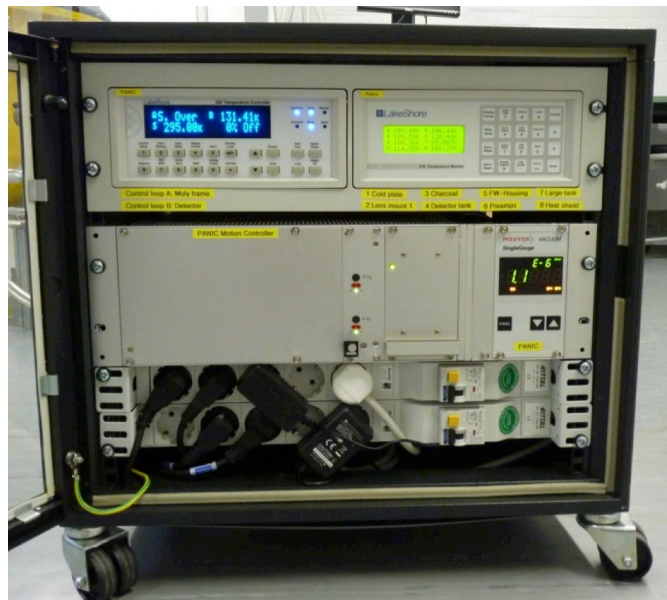
Figure 3: Control electronics rack. Top row left: Detector thermal control, right: temperature monitor. Center row left: MPIA motion controller, right: Pressure gauge. Bottom: Power supply and fuses. Mounted on the rear side are the Ethernet switch and Nport server.
